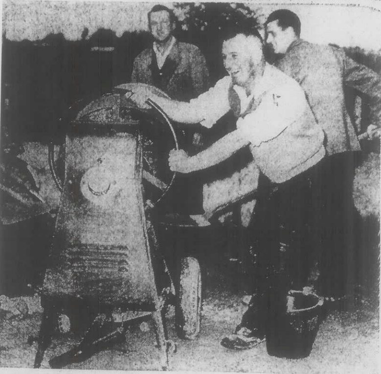
(right) gives a helping hand to the Young Munster men at the erection of the new pavilion at the Young Munster Grounds at Rosbrien.
