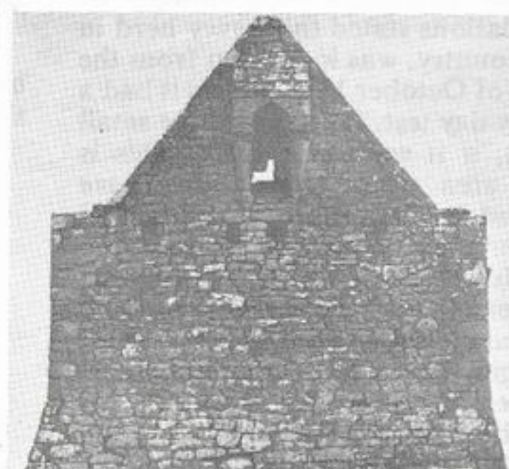
KILLEEN: West gable with pronounced wall batter and turret-like belfry on corbels.
