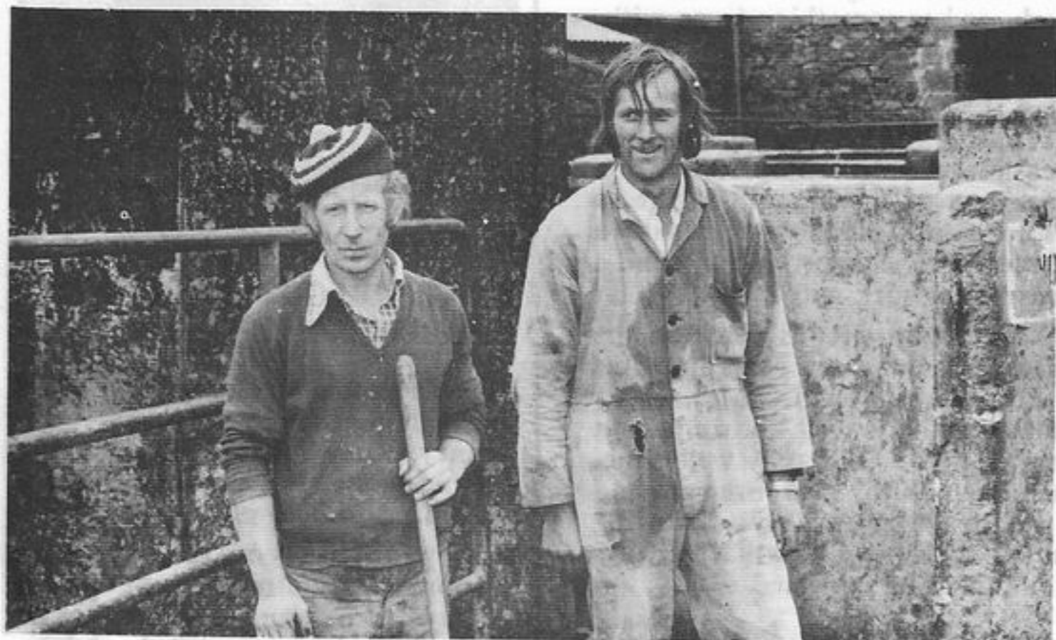
Busy covering the Lairage area are John Sheahan and Pat O'Connor of Nash's Construction.
