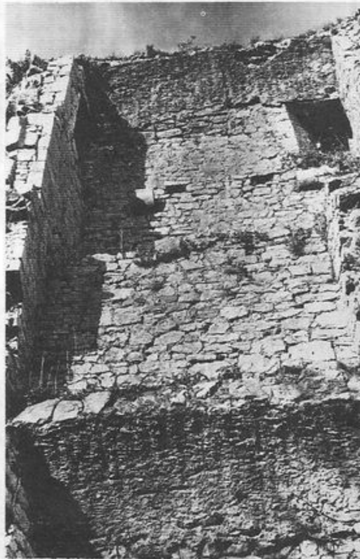
Garraunboy : Corbels for floor joists. Note wicker impressions on mortar under floor vaults. [Photo : Author].
