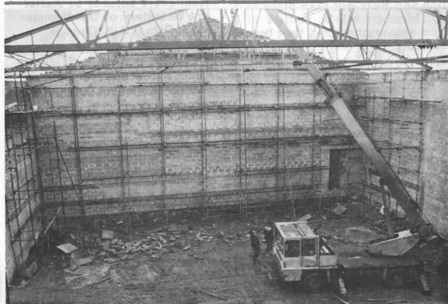
The new Cold Store takes shape. The above photograph gives an indication of the dimensions of the new building which will be in use within a short period.
