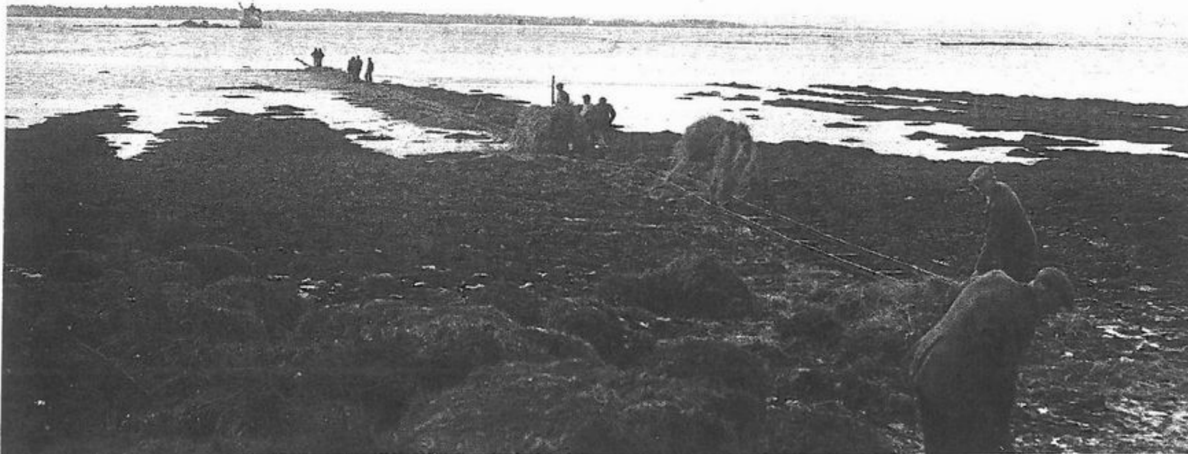
Board of Works employees and volunteers laying a temporary railway line from the shoreline to the site of fatal crash at Shannon, 10 September 1961. The rails were used to trolley wreckage and debris from the site. The hay was placed beneath the rails to prevent them sinking in the mud
