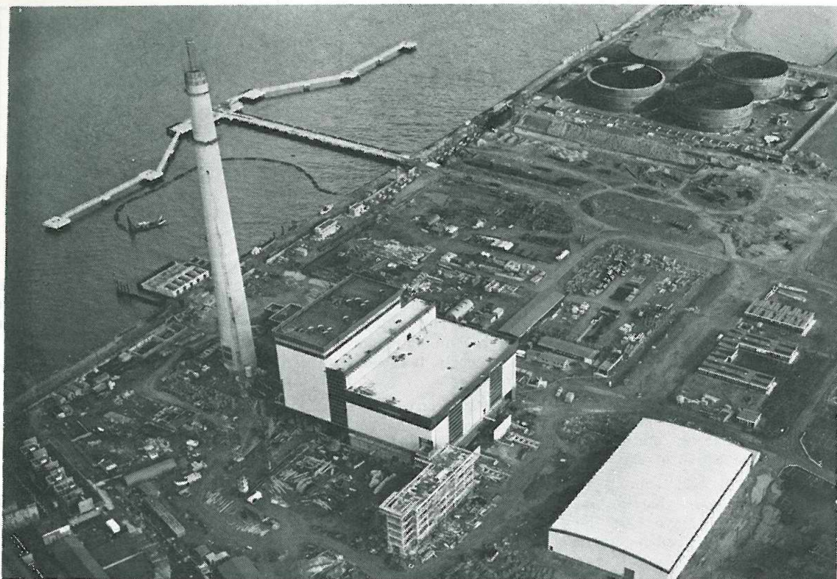
The E.S.B. Pigeon House 'B' generating station now under construction at Ringsend in Dublin
